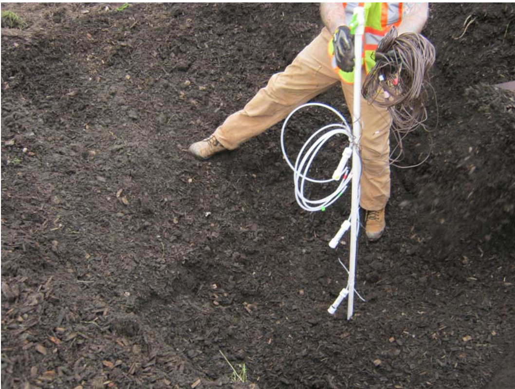
Figure 3. Installation of the monitoring equipment at the Clearwater biofilter.
