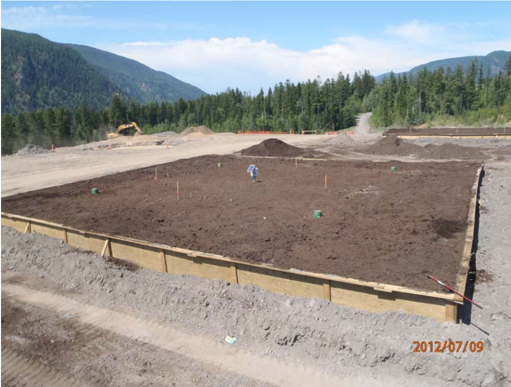
Figure 4. Clearwater biofilter surface after installation of the monitoring equipment.
