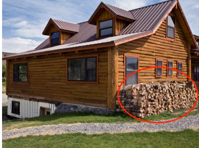
Figure 9 Firewood stacked within 10m of the home during wildfire season poses a significant threat to home ignition and therefore should be stored outside of PZ-1 (photo not taken from Loon Lake)
