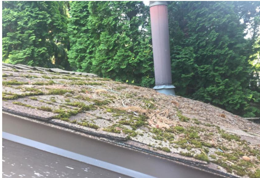
Figure 7 Combustible debris (organics) pose a risk to home ignition as they can challenge the roof materials resistance to fire. As well, aging roofing material poses a risk to exposure of combustible wood underside (photo not taken from Loon Lake)
