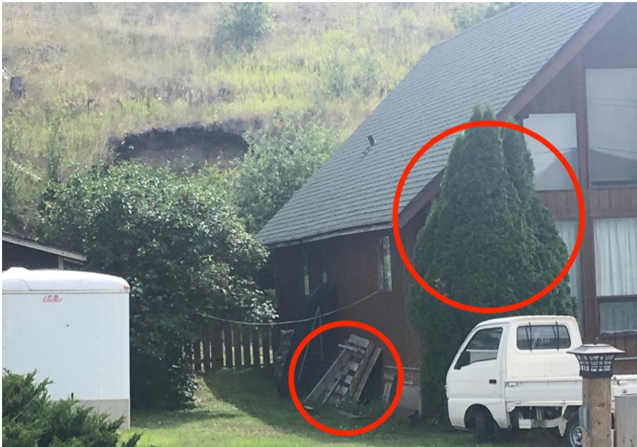
Figure 8 The presence of nearby combustible debris (such as wood pallets, ladders, building materials etc.) and combustible plants pose a high risk to ignition of a building's exterior. (photo not taken from Loon lake)
