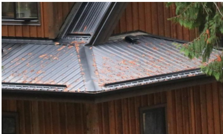
Figure 9 Roofs that are free and clear of debris help to mitigate the risk of home ignition
