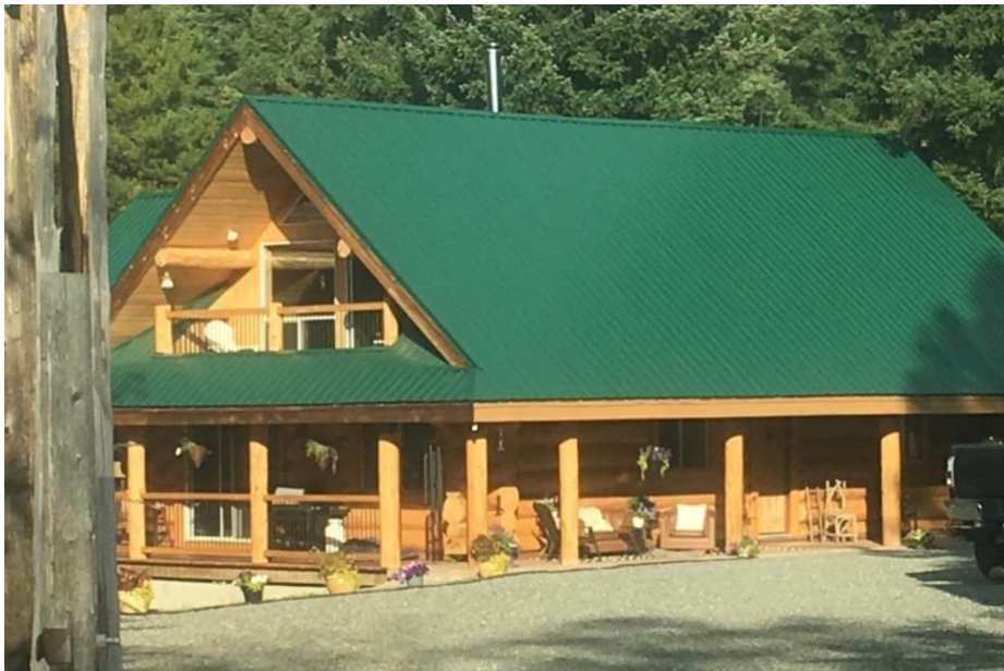
Figure 9 Fire-rated roofing material is proven to be highly resilient against home ignition during a wildfire event. Roof design can also contribute to mitigation of debris accumulation by minimizing valleys and pinch point where debris can be captured
