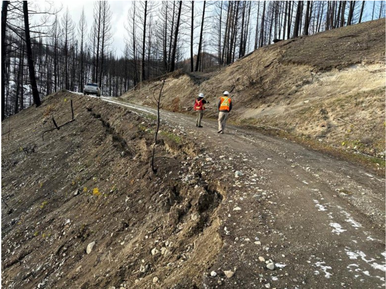
Photo D-35 Looking north along Twaal Creek Rd and landslide at the road. Photo taken by BGC on November 18, 2024.
